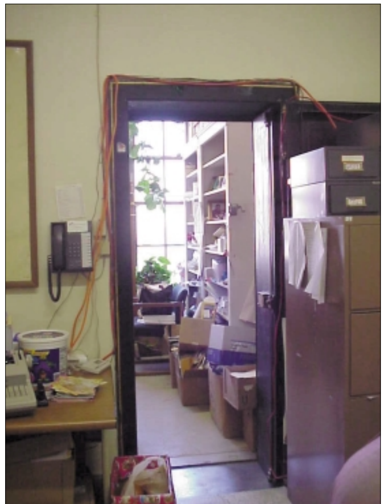
Detail of computer wiring, Room 112
