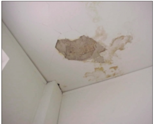
Damage to ceiling, District Clerk's Administrative Office, Room 210
