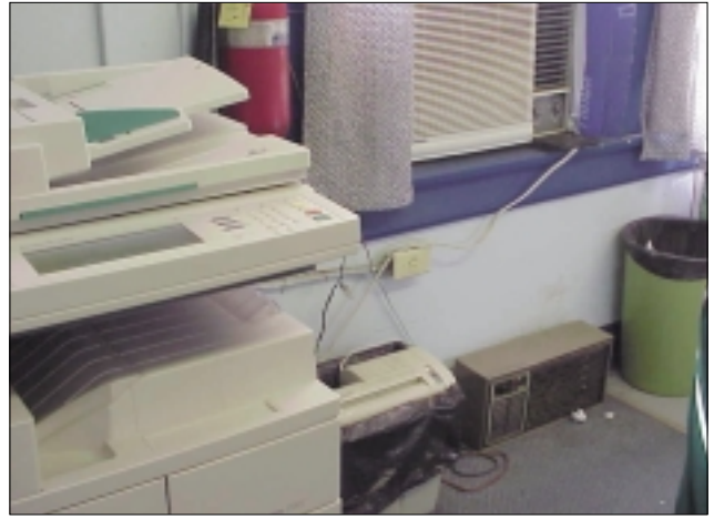
Detail of wiring in Sheriff's Dispatch Office, Room 212
