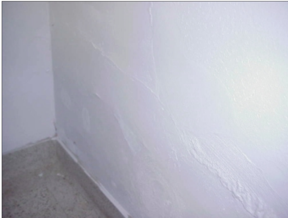
Detail of damaged plaster, Room 105
