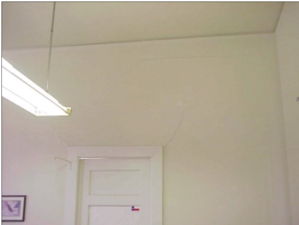
Cracked plaster, Room 102
