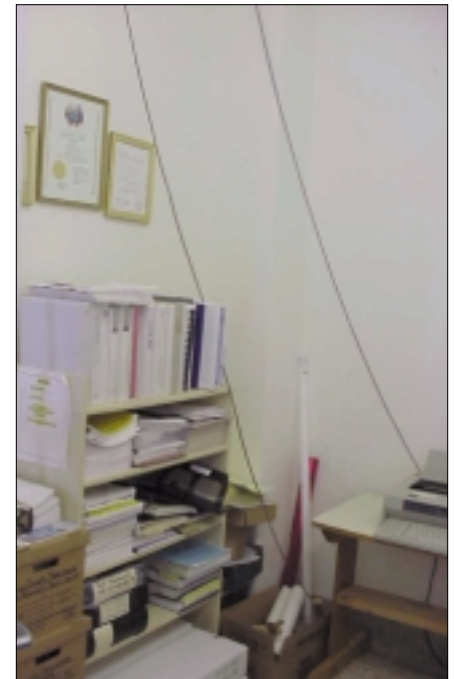
Detail of extension cords, through wall to adjacent room, Room 109
