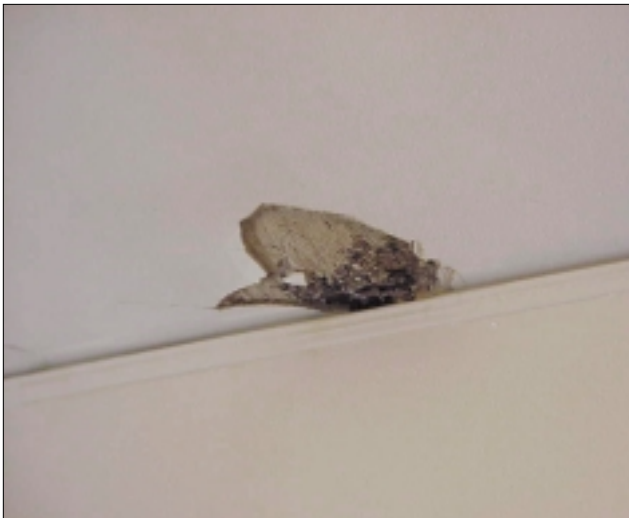
Ceiling damage in corridore, Room 206
