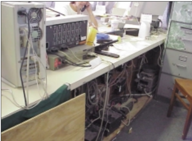
Detail of wiring in Room 212
