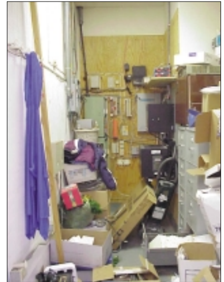
View into 911 mechanical and telephone room, Room 213
