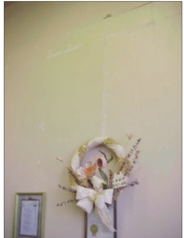
Cracked plaster, Room 111
